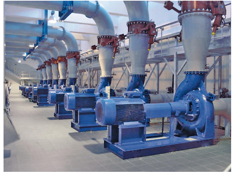
Boswell & SWP Pump Stations
