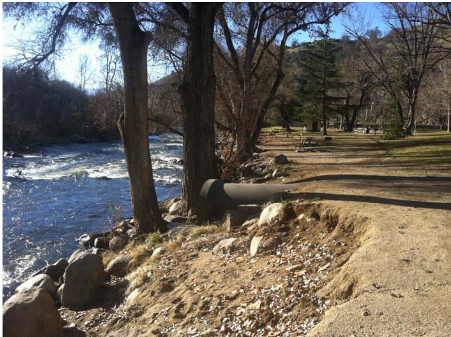
Figure 10: Erosion at Riverfront Park
