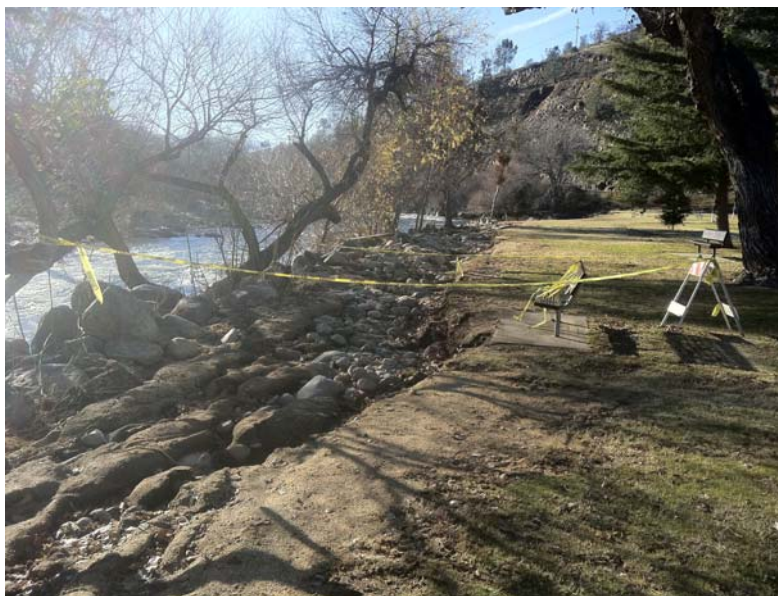
Figure 12: Degradation associated with flooding
