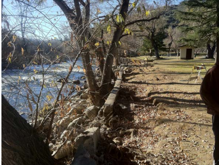
Figure 11: Erosion and degradation of longitudinal floodwall
