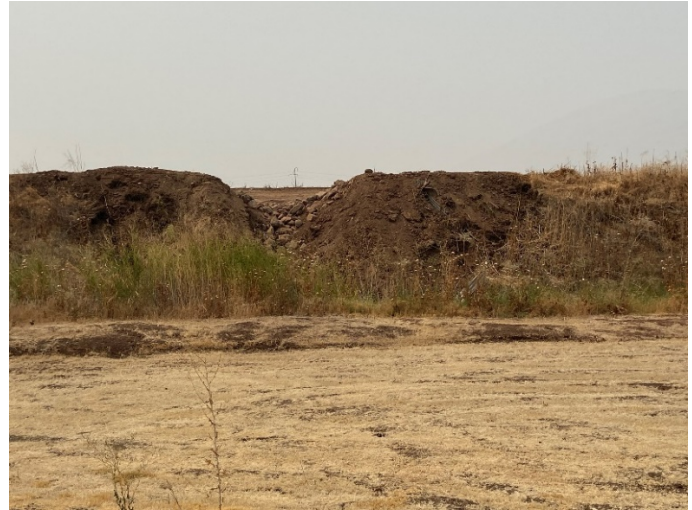
Embankment was cut out and armored with rock to allow runoff and minimize erosion.
